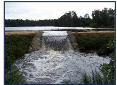
This dam failure caused flooding that damaged several homes and vehicles.
